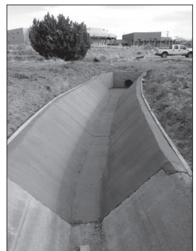
Crews from the Natural Resources Department and Public Works helped repair ditches damaged in an autumn storm to prepare them for the annual Ditch Work project in March. Photo by Greg Kaufman, NRD Director
